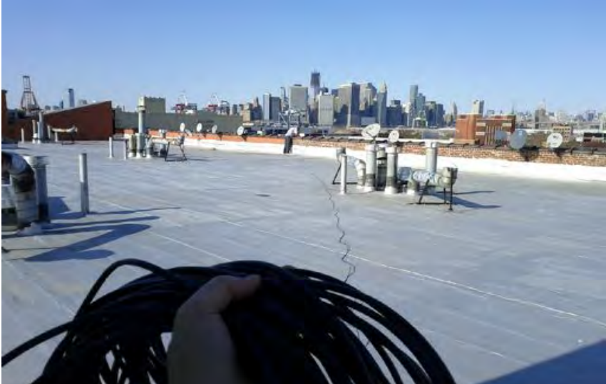
Figure CsOTI 5: Running cable to install a node on the roof of an apartment building north of Coffey Park.
