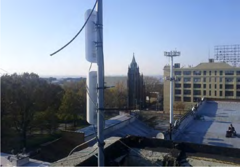
Figure CsOTI 14: Rooftop node installed after Superstorm Sandy.
