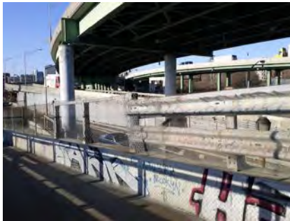
Figure CsOTI 3: Gowanus Expressway which divides the Red Hook neighborhood from the rest of Brooklyn.
